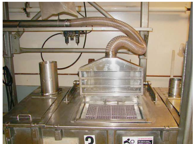
Slotted backdraft hood behind grated inlet of dumping station. All hoods are made of food grade 304 SS.
